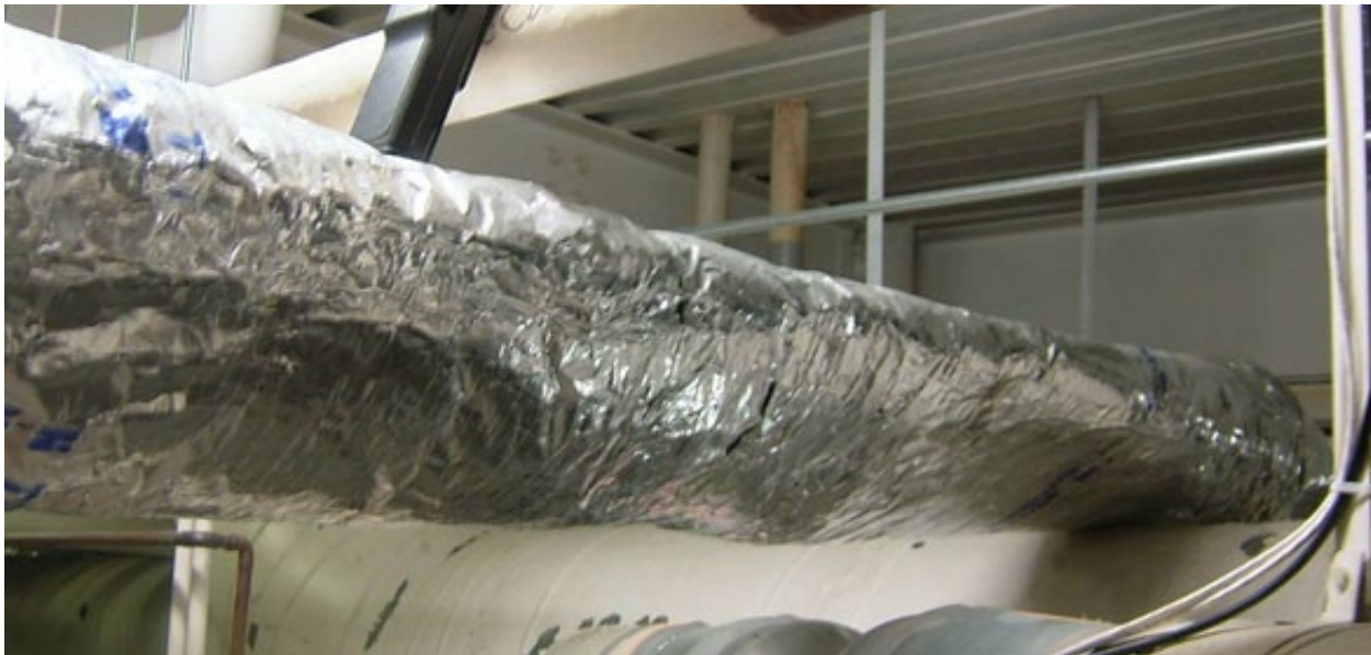
Fig 3 – (Exhaust duct implosion when room bubble tight damper tripped closed)
